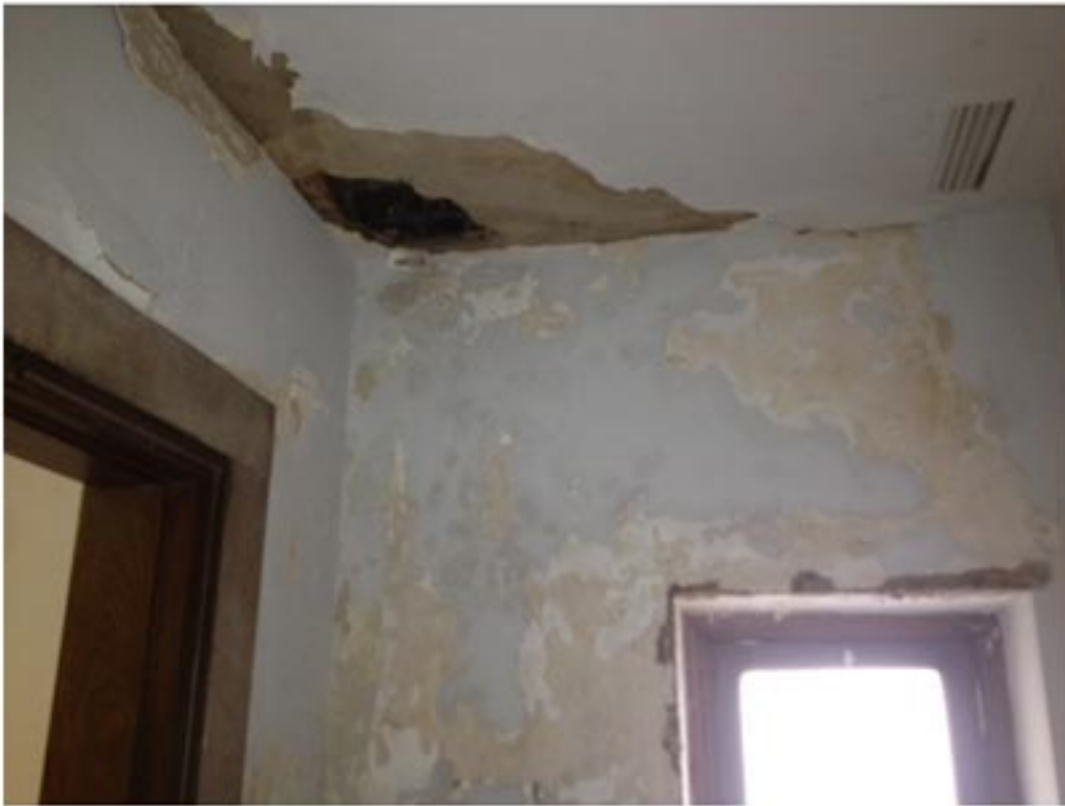
Third floor bathroom, southside of building. Photo shows intrusive water damage.
