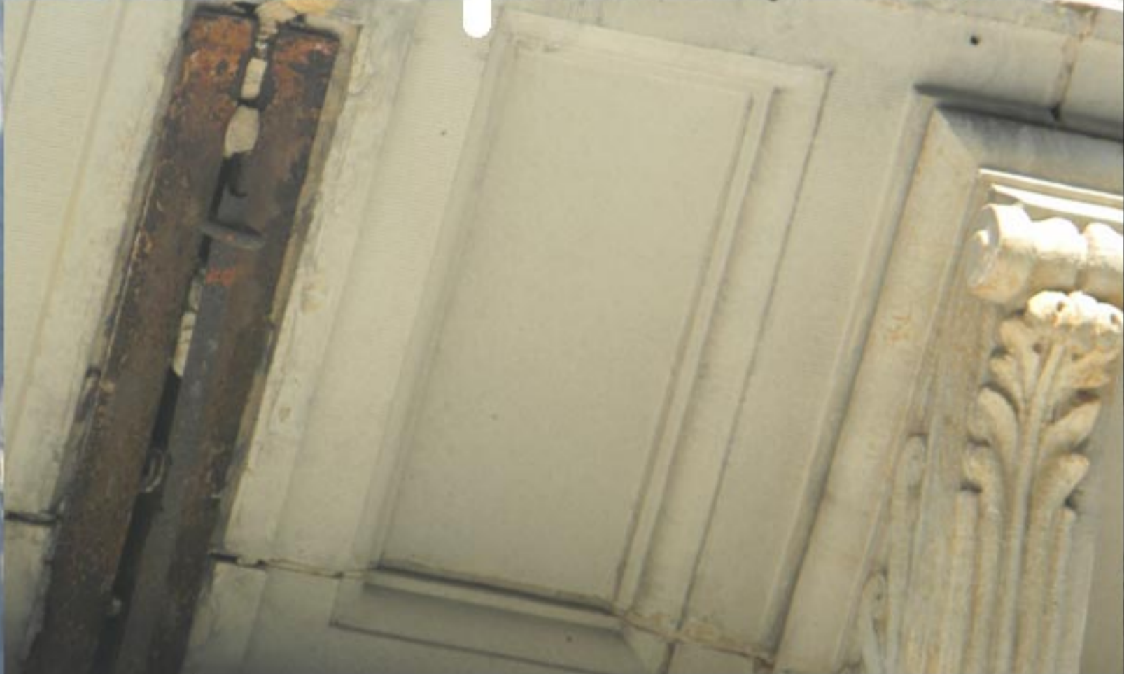
FALLEN CORBEL, CORBEL CRACKED AND FELL TO GROUND.
