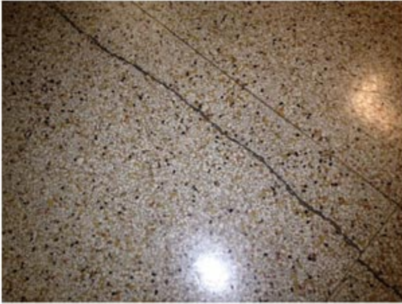
Major floor crack which runs perpendicular to the support wall of the Bell Tower. The Bell Tower also has cracks.
